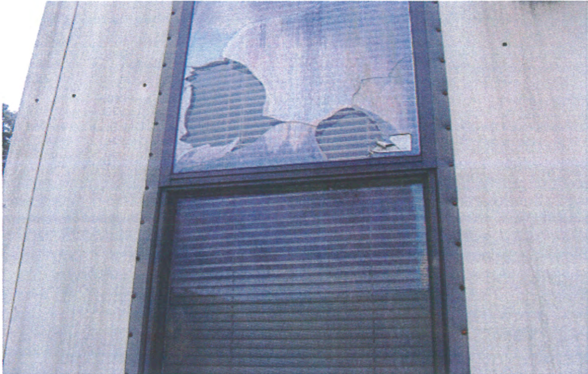
View of Vandalism ↑
