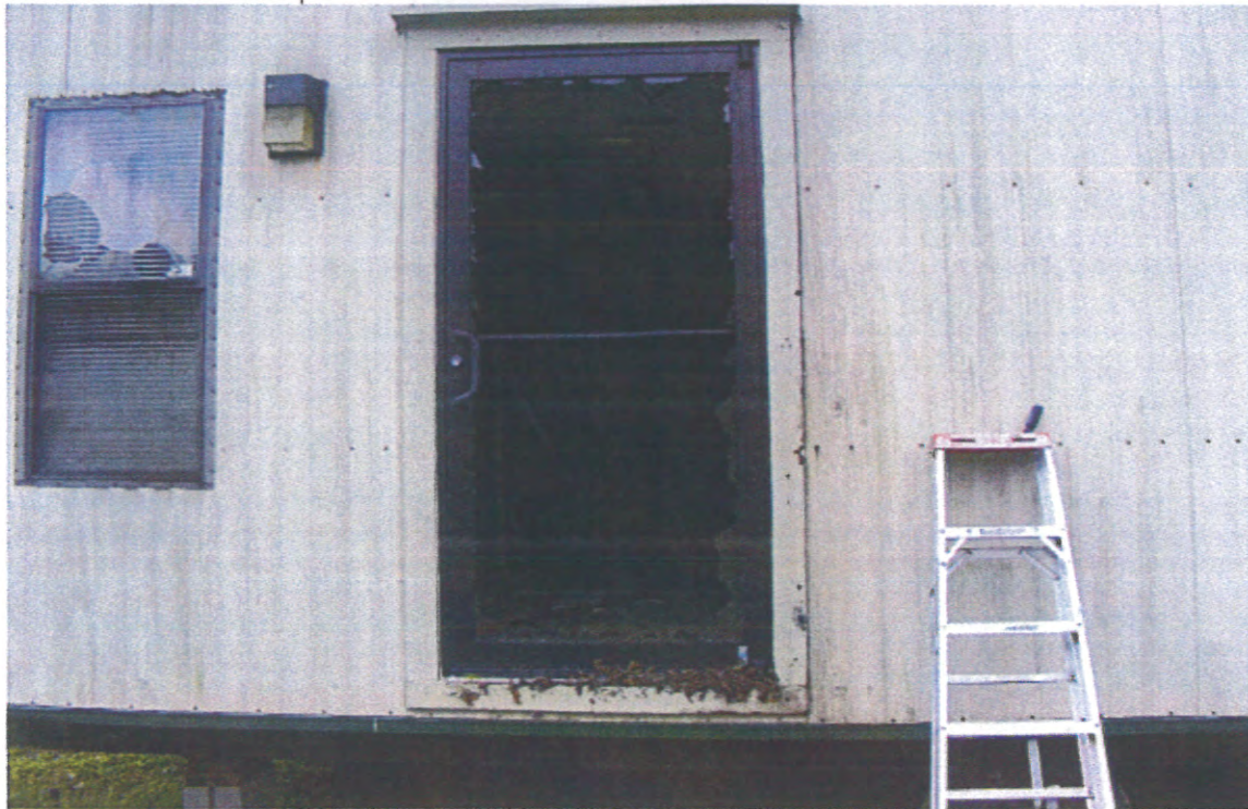
View of Vandalism ↑
